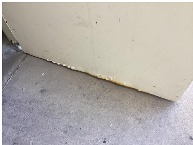
Door rust at building 7 trash room
