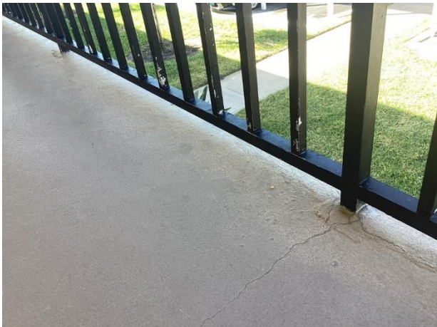
Cracks and previous repairs at breezeway railing posts
