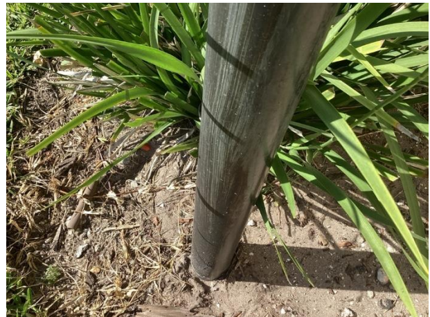
Finish deterioration at light pole
