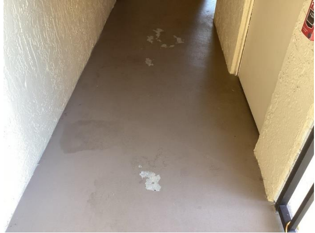
Coating delamination by unit 4207
