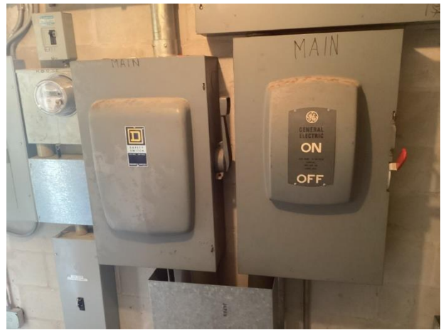
Electrical system main panels
