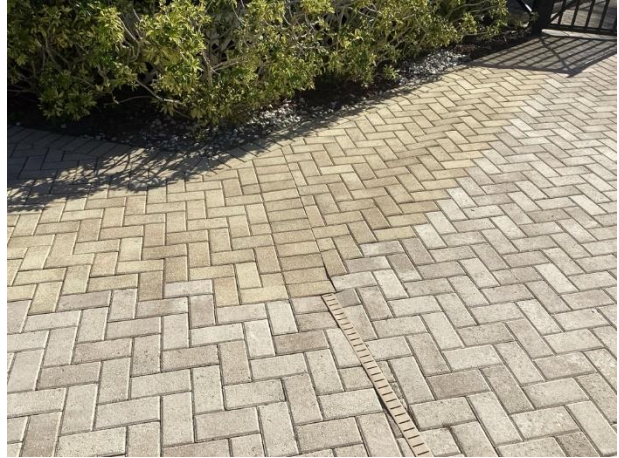
Previous paver repairs
