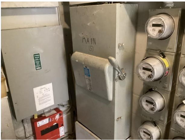
Electrical system main panel
