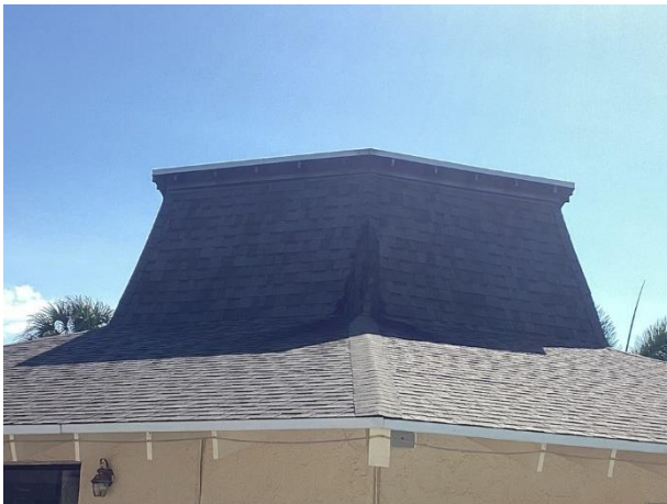
Clubhouse roof with worn shingles
