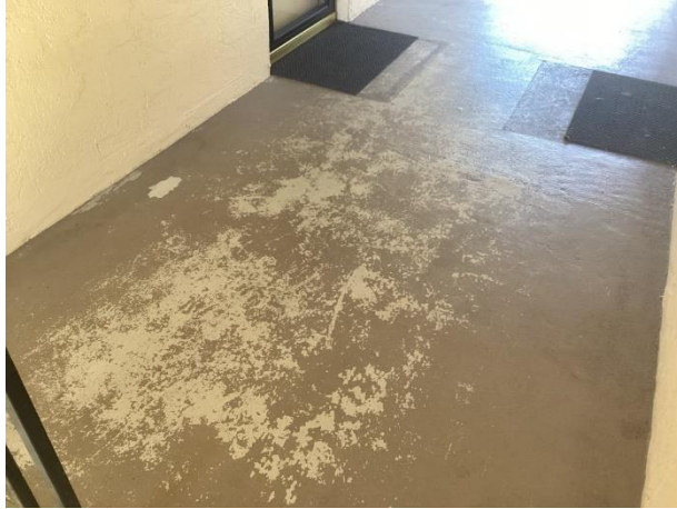
Delamination by unit 3206
