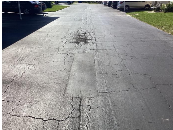
Pavement overview with cracks and patches
