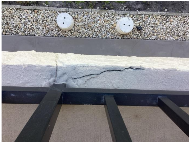
Concrete edge cracks by unit 8206
