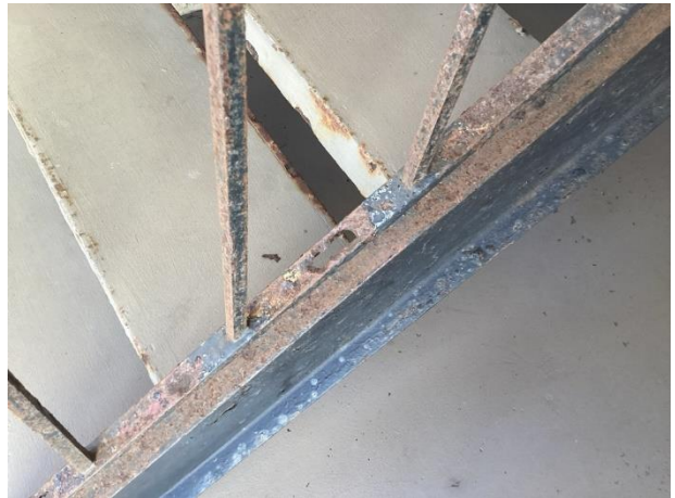
Rusted through railing at unit 3106
