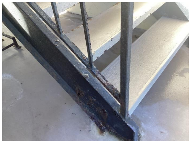
Staircase rust by unit 2101
