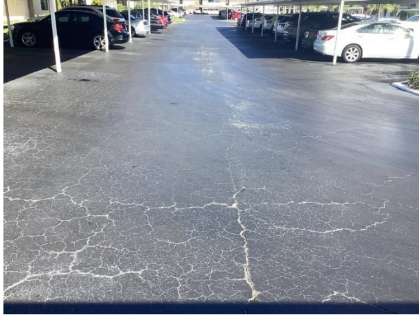
Pavement with cracks
