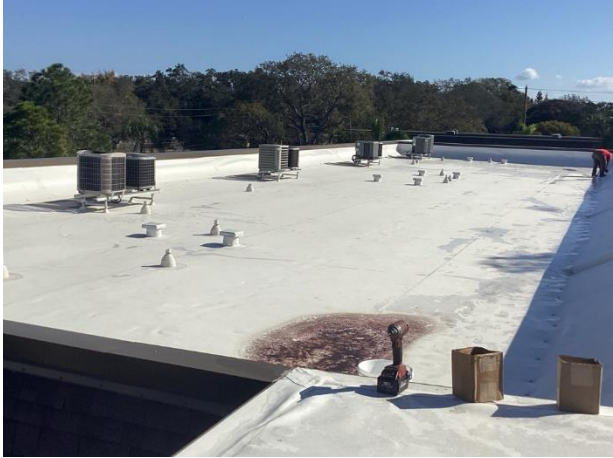
Roof with isolated area of standing water
