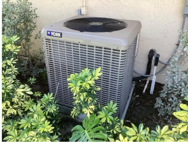
Split system condenser at clubhouse
