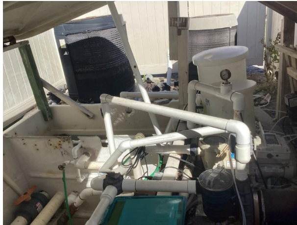
Pool mechanical equipment
