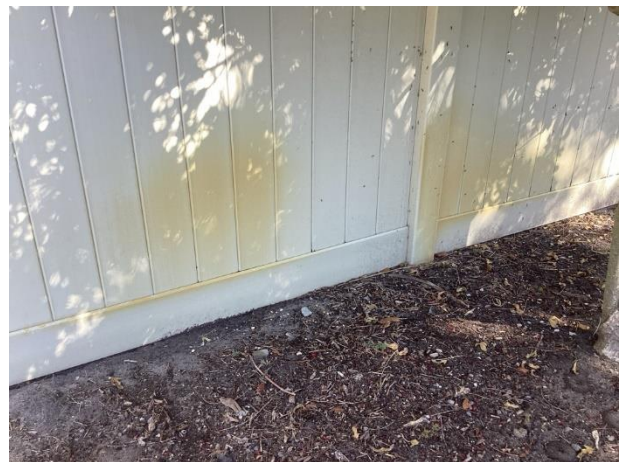
Stains at perimeter vinyl fence
