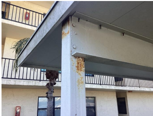
Rust at old carport post
