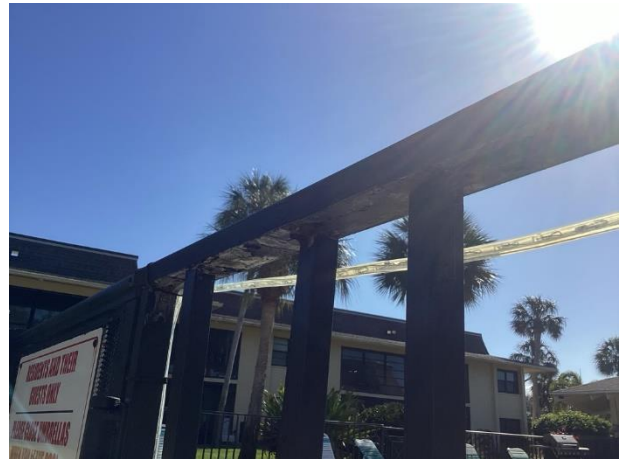
Fence damage and previous repair
