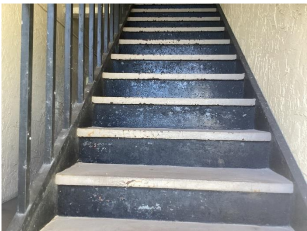
Staircase with rust by unit 8101
