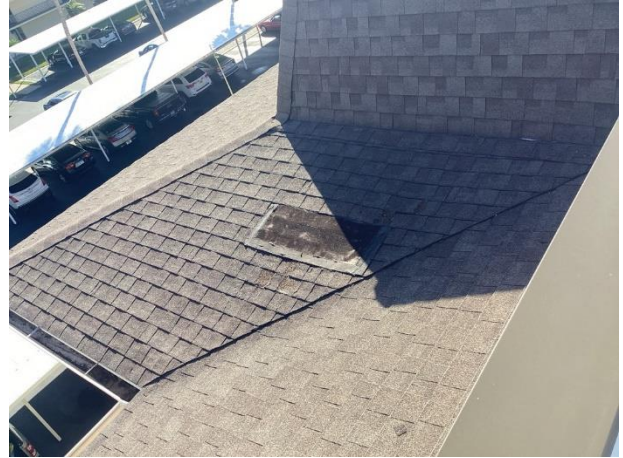
Missing shingles at building 5
