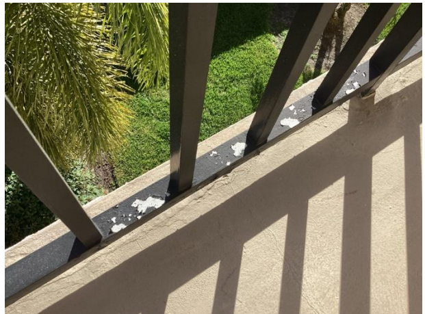
Peeling paint finish at breezeway
