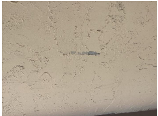
Stucco damage at unit 1102
