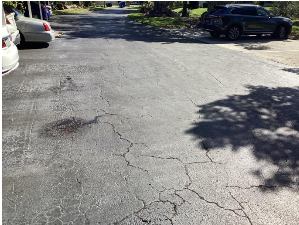
Pavement with cracks
