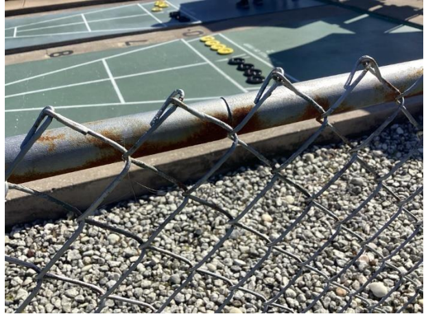
Fence pole rust
