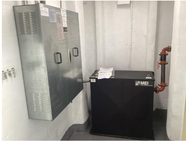
Hydraulic elevator equipment
