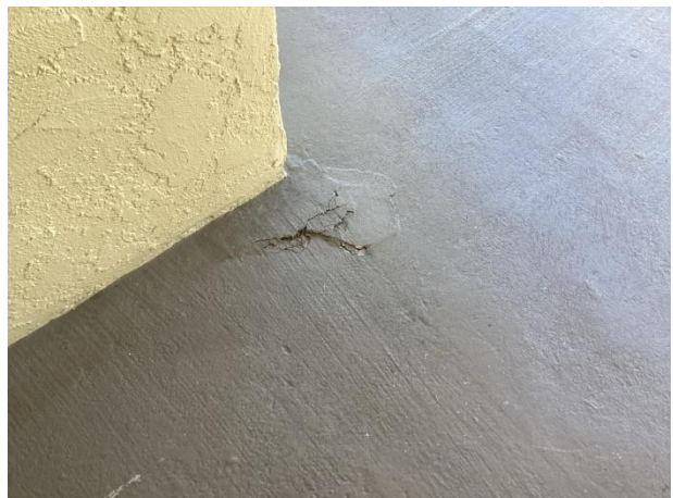
Concrete damage by unit 3201
