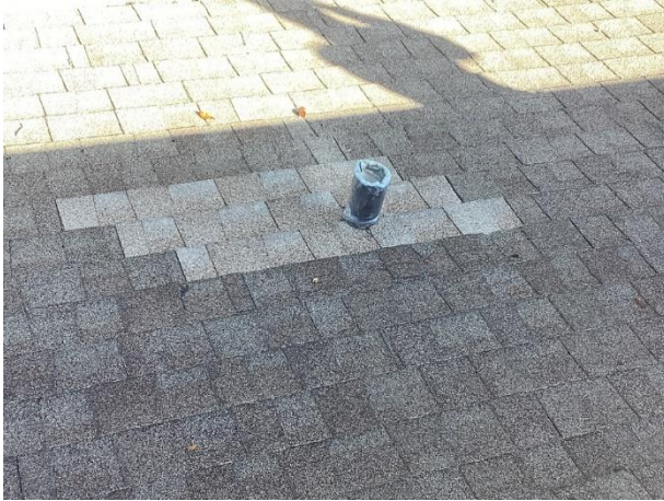
Previous repair at roof penetration
