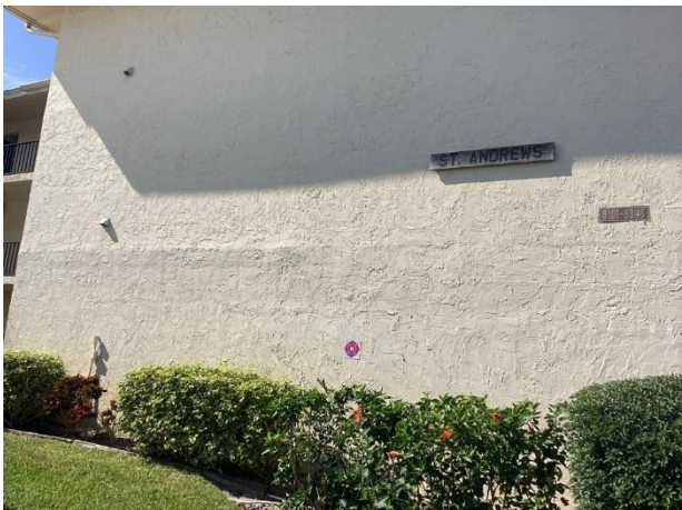
Evidence of potential moisture intrusion
